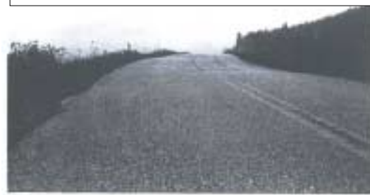
Flexible Pavement Low Severity
