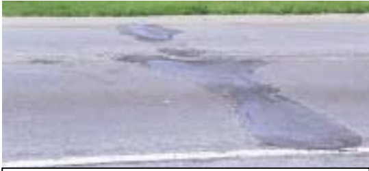
Flexible Pavement High Severity Patching
