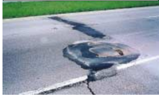
Composite Pavement High Severity
