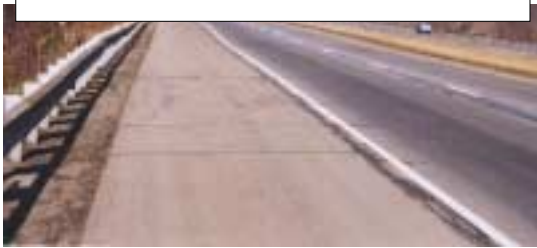
Composite Pavement Medium Severity
