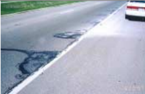
Composite Pavement Medium Severity
